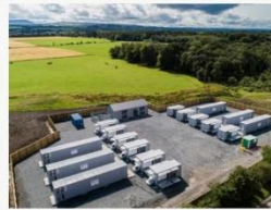
Braxburn Energy Storage System, West Lothian © Keith Atkins
