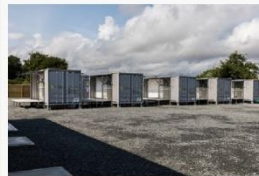
Braxburn Energy Storage System, West Lothian © Keith Atkins
